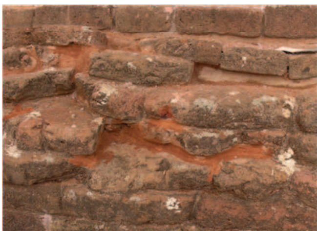
Figure 4. Mortar used in the square chamber of Jethawana sthupa (reddish colour area is the mortar which is used for the conservation).
